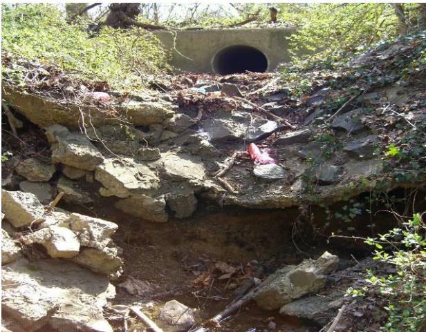
Figure 4-9: An eroded outfall
