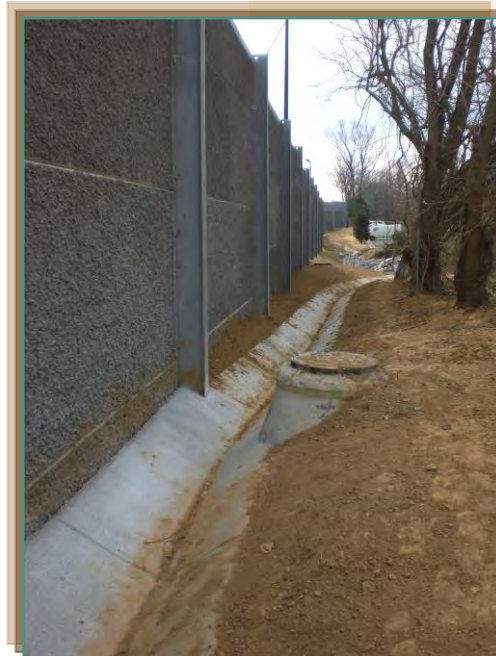
Sound wall and drainage ditch along eastern side of Hartland Green Park
